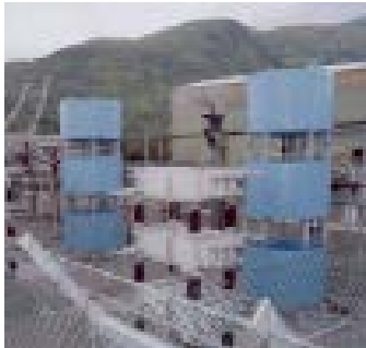
Figure E.6.1 Air core reactors (blue), image courtesy of Enspec Power
