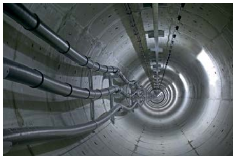
Figure E.2.1 Transmission cables installed in a 4m tunnel
