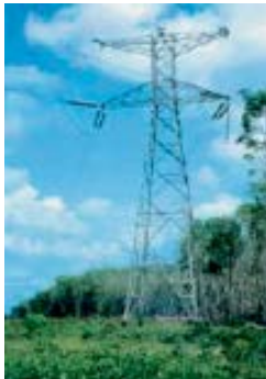
Figure E.20.1 Bipolar tower 300kV link Photo courtesy of Siemens
