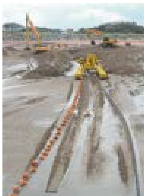
Figure E.3.3 Cable plough on shore. Image courtesy of IHC Engineering Business.
