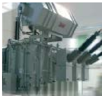
Figure E.5.1 Power Transformer
