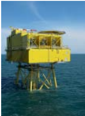
Figure E.17.1 BorWin1 HVDC platform, North Sea. Image courtesy of ABB.
