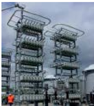
Figure E.7.1 National Grid 275kV capacitor bank
