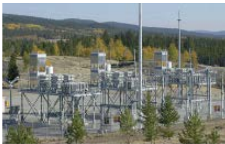
Figure E.10.1 Series compensation installation (courtesy of Nokian Capacitors)
